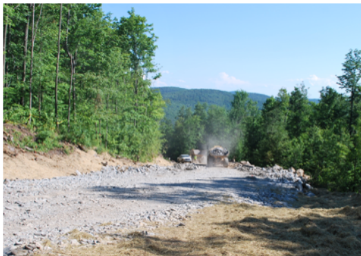
J.A. McDonald, site constructors working on the Project access road in early July.
